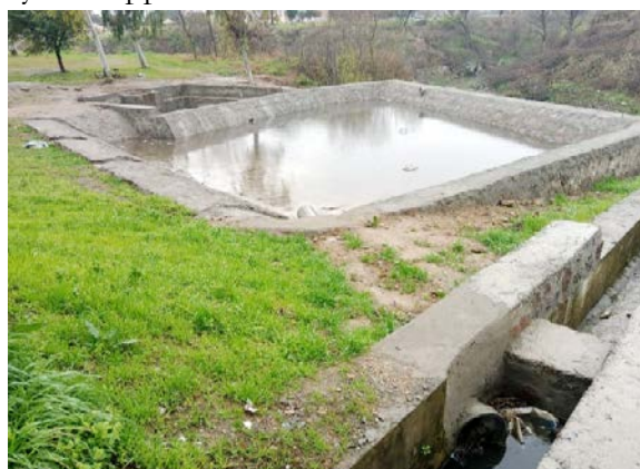
Figure 3. Rainwater harvesting in parks
